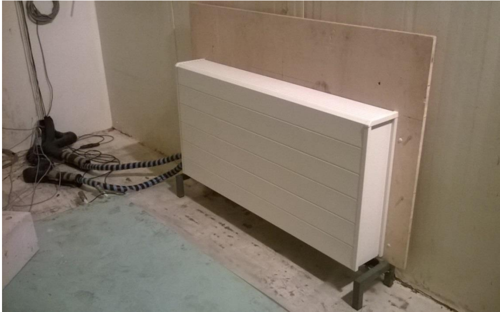
Foto 2.4 Low-H 2 O radiator in de proefkamer
